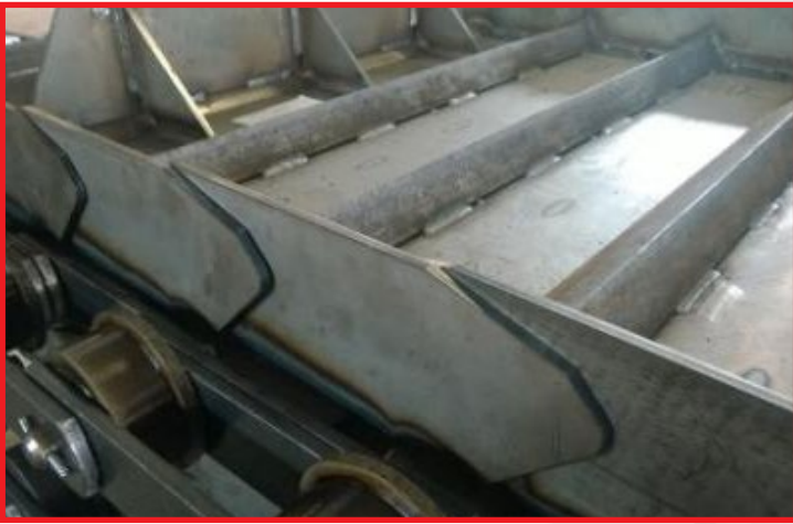
Waste combustion plant
